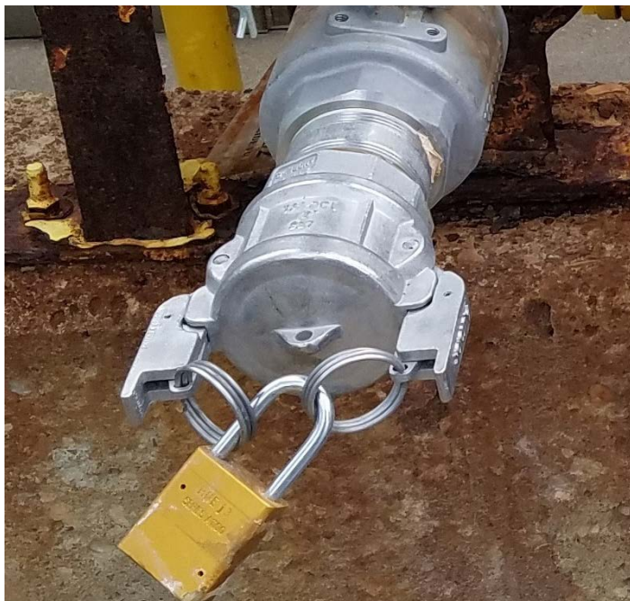
Figure 5. A locked cam lever dust cap on a fill line at Mod B (Source: CSB).
